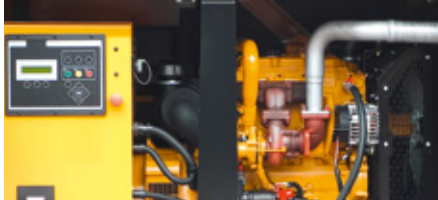
Mobile power generation
